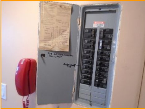
Gould Electrical Panel
