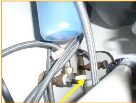
Missing Shut Off Handle
