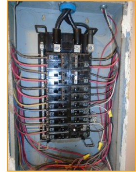
Gould Electrical Panel Wiring
