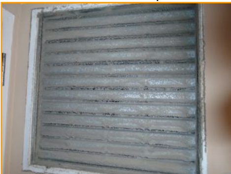
Dirty Heat Pump Coils
